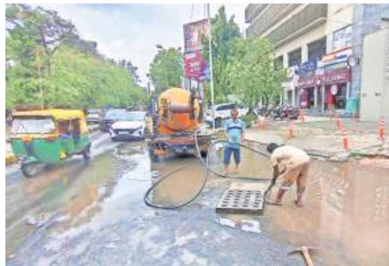
Maintenance work in progress to declog drainage line at SV Desai Marg in Navrangpura on Sunday. Nirmal Harindran
